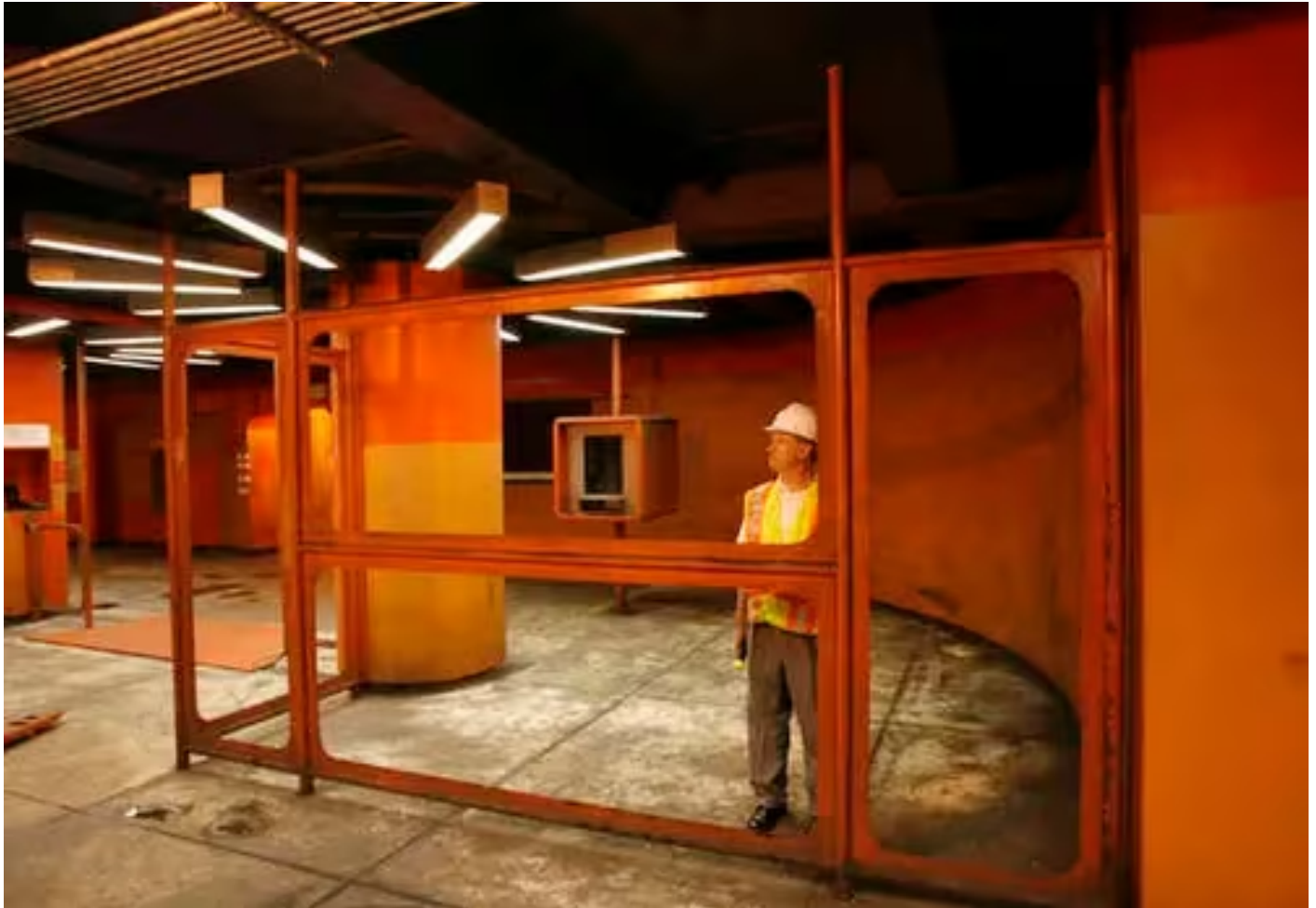
The 1970s orange fare collection area in the closed Franklin Square Station gets a once over in 2007 from John Matheussen, then chief executive of the DRPA.
