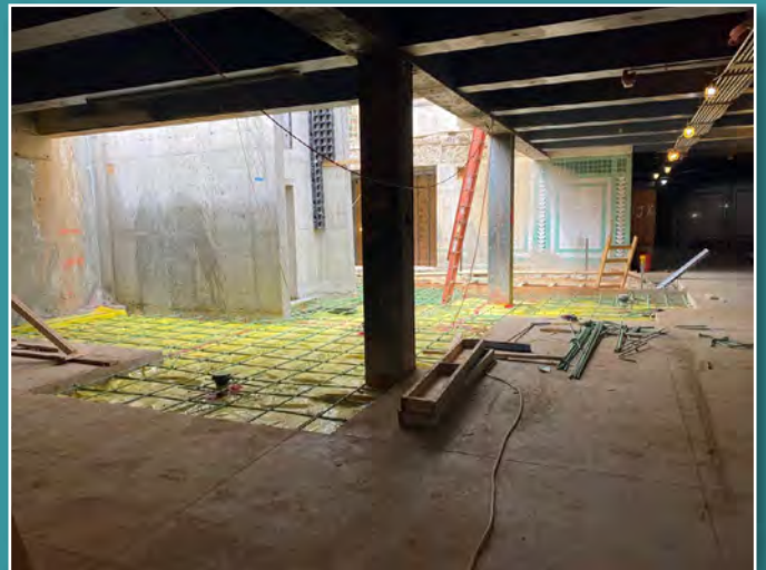
The concourse level floor slab has now been constructed at the base of the entrance staircase and elevator.
