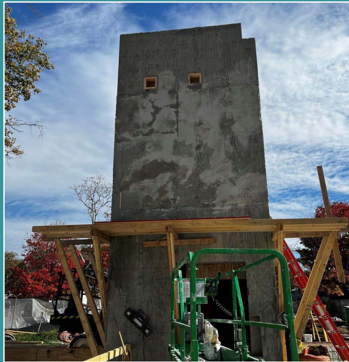
Concrete has been placed for the last segment of the elevator shaft.
